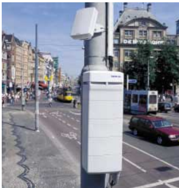
3G auction could speed up deployment of cellular infrastructure.
