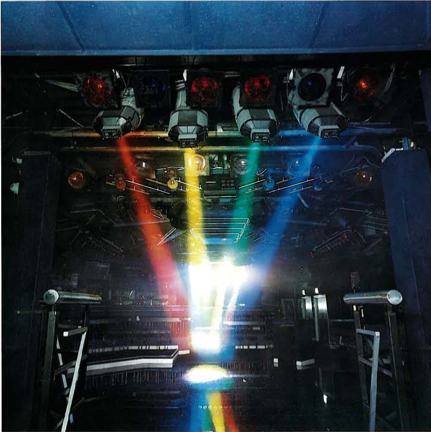
A close-up of the first UK installation of Clay Paky Golden Scans.
